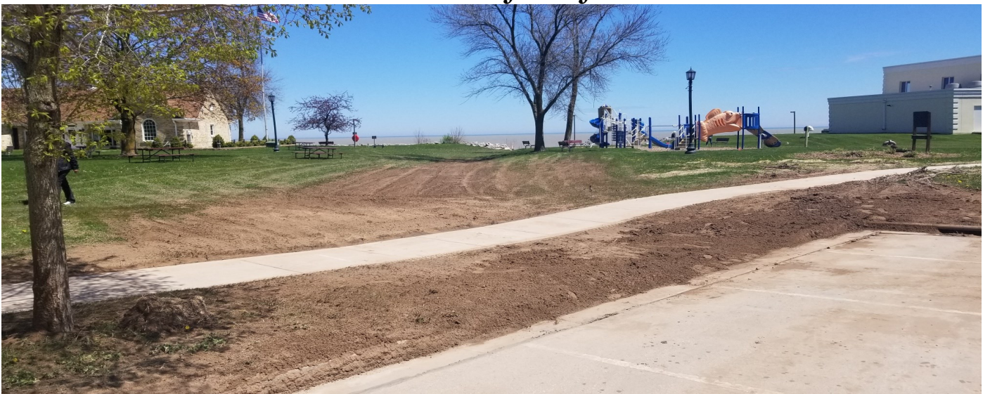
Veterans Park flood restoration
