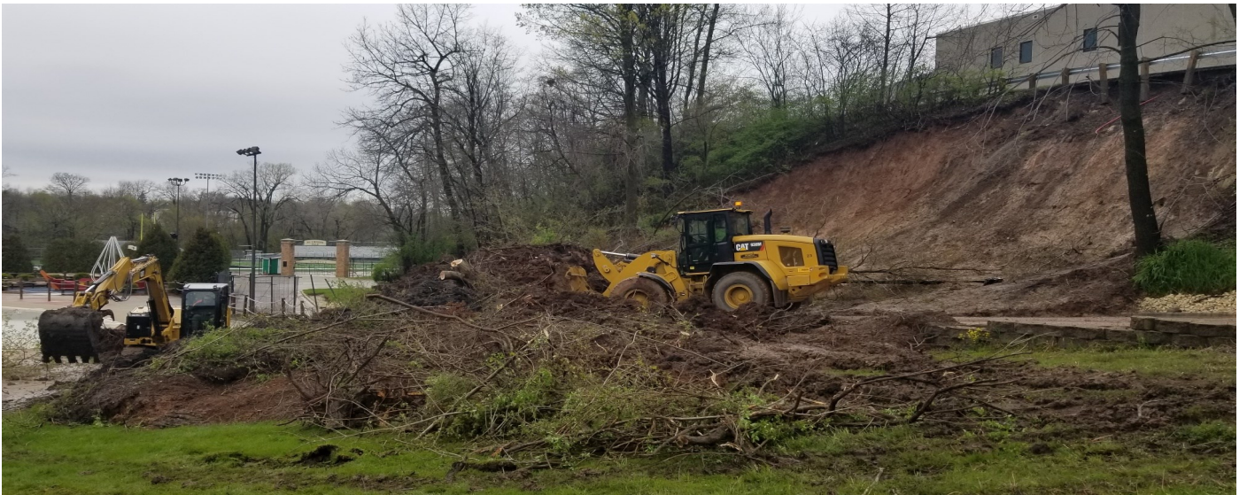
Debris Removal from flood
