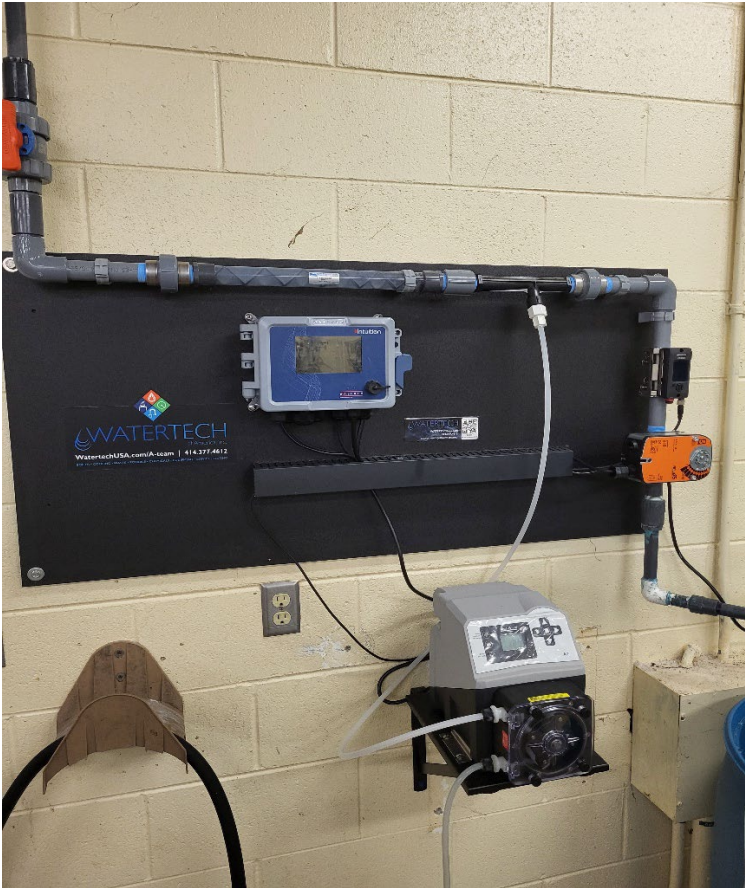
Figure 2- New polymer make-down unit for digested sludge.
