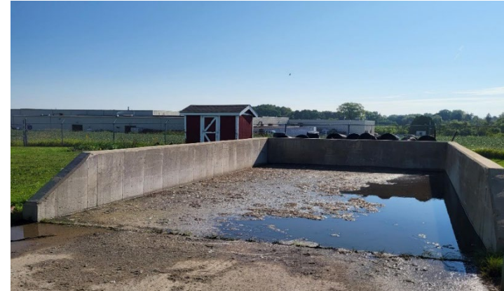
Figure 2-Remote Site Drying Bed
