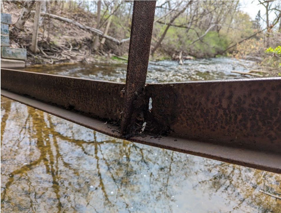
Photo 5. Lower arch connection damage
