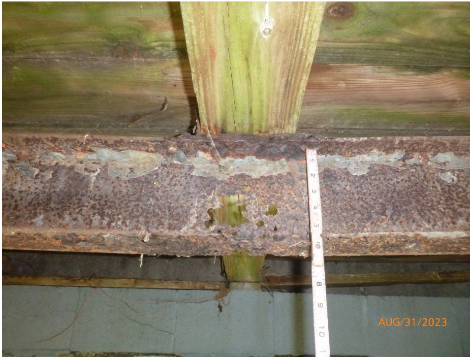
Photo 4. Cross bracing damage
