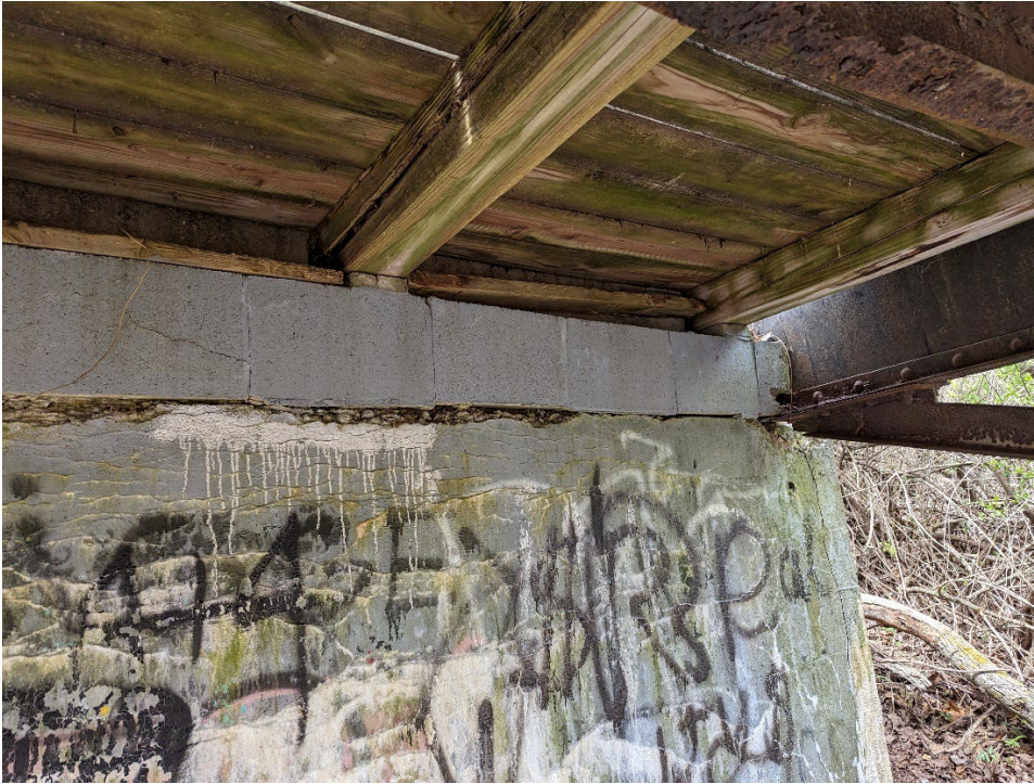
Photo 1. Longitudinal stringer damage west end center
